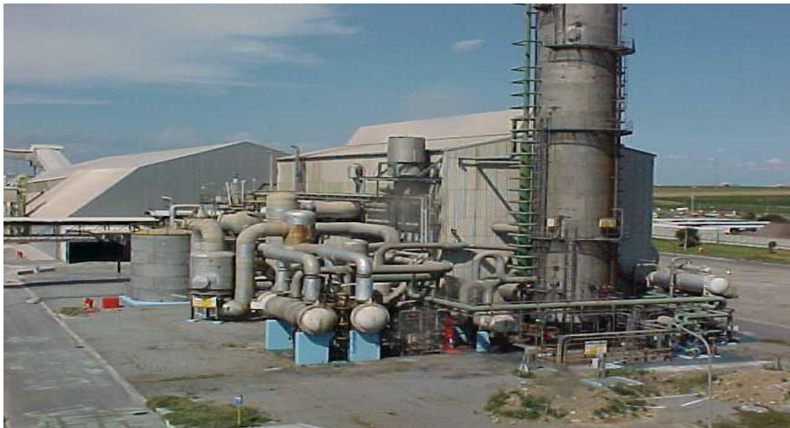
Figure 10. Sasol Nitro Nitric Acid Plant, Sasolburg
